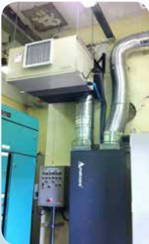
AIRWASH 10 000 PETRO CHEMICAL FACILITY
